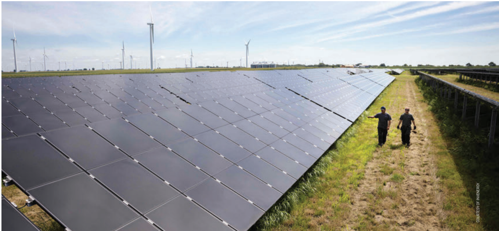
Megawatt mega-walk. Some of Invenery's projects are quite sizeable, such as the Grand Ridge Solar Farm near Streator, Ill., the largest solar farm in the Midwest when it was built in 2012.
