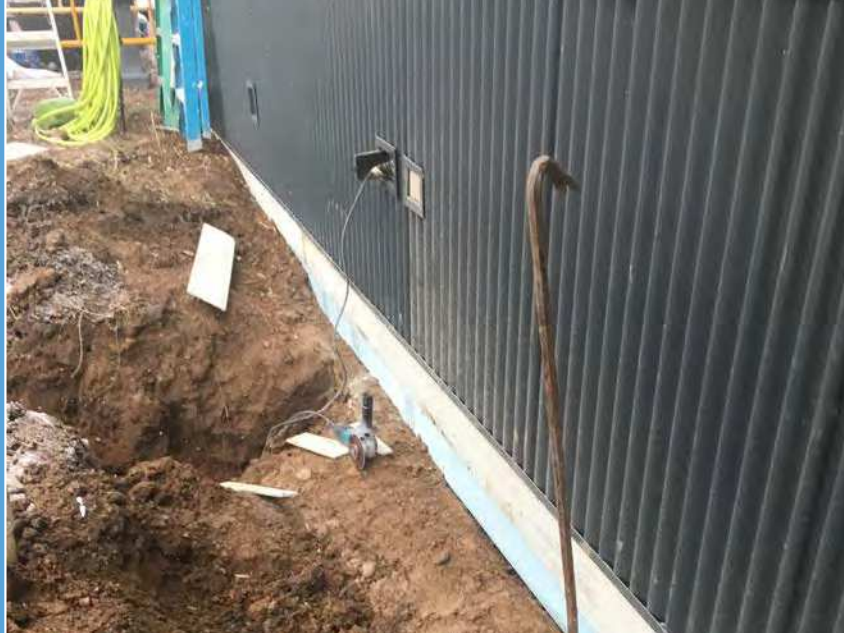
Plumbing and electrical systems for the barn, which has been inhabited for 16 years, did not meet code and had to be replaced. The perimeter insulation also decreased 1.6 inches by using R-5 rigid.
