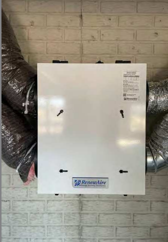
Air equality. The VISION House features balanced ventilation supplied by a RenewAir energy recovery ventilator.
