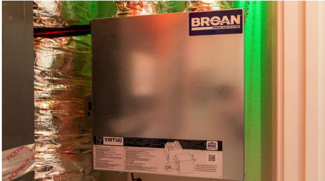
A winning team. Indoor air quality is enhanced with Broan-NuTone’s ERV and its Evolve continuous run exhaust fan, which automatically monitor and clean the air. CREDIT: GREEN BUILDER MEDIA/SAMANTHA CARLIN
