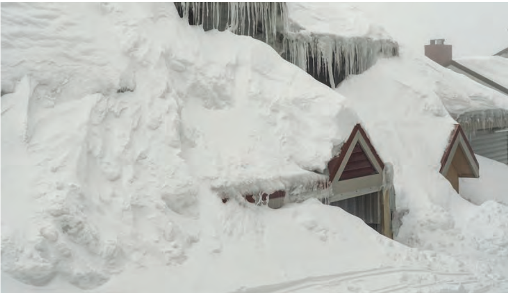
Ready for this? Super-insulated housing envelopes offer a hedge against extended power outages in extreme conditions. CREDIT: ISTOCK/CHRIS GORDON
