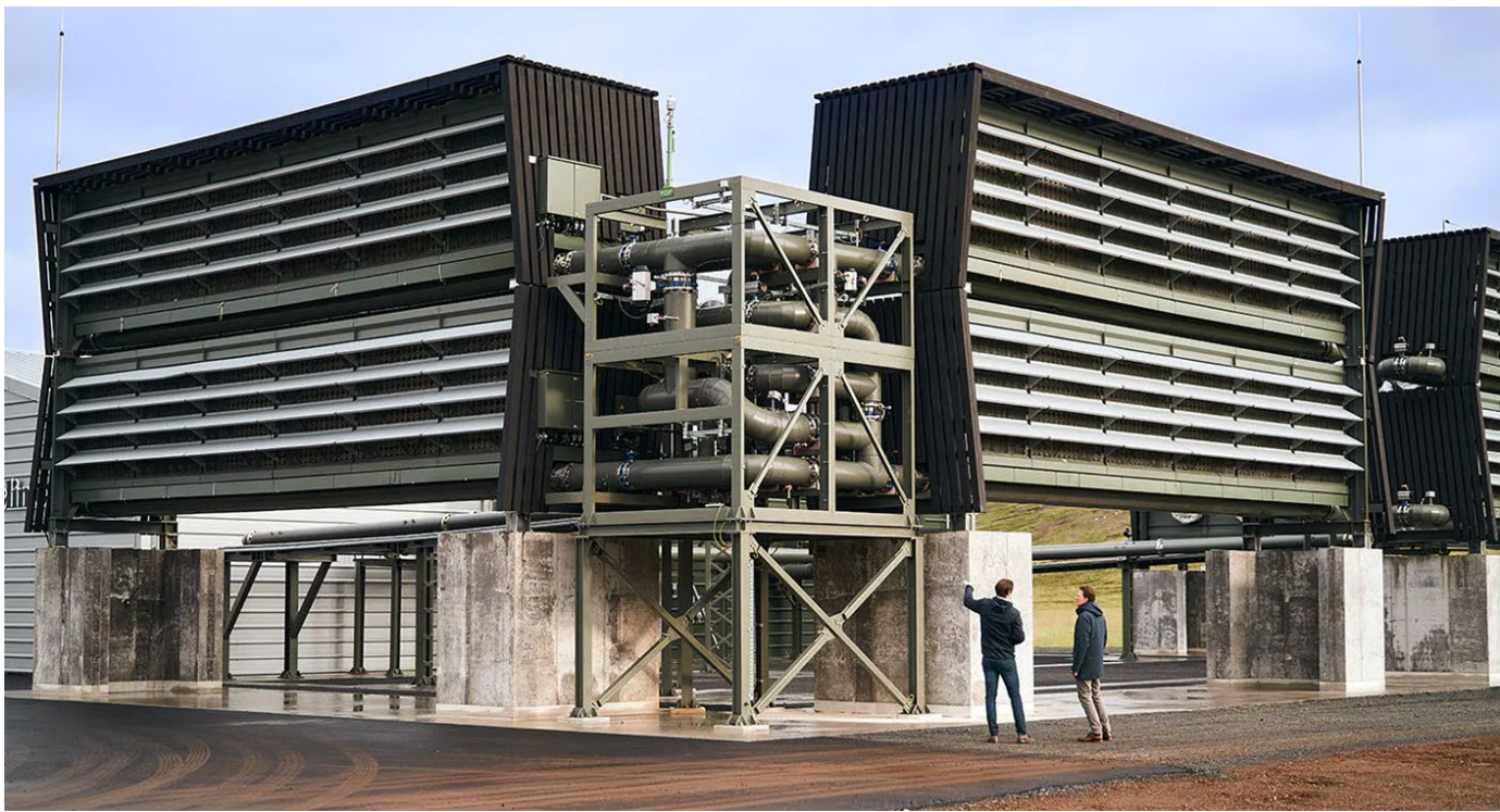
Air scrubber. Orca is the world's largest direct air capture plant, capable of eliminating 4,000 tons of CO 2 from the atmosphere each year. It's also aptly named: "Orca" is the Swiss word for "energy." COURTESY OF CLIMEWORKS
